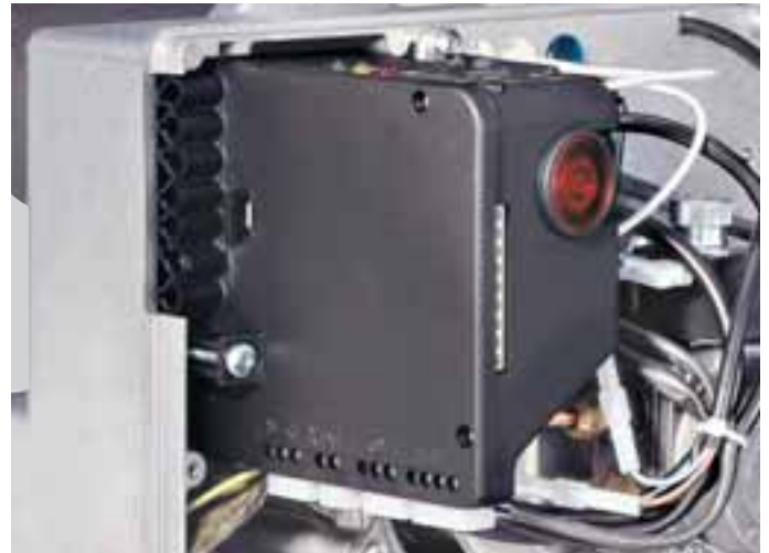
Control box fitted with ignition transformer
